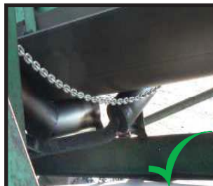
The 6mm galvanised chain installed to hang at the same curve as the conveyor.
